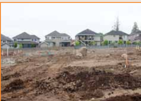
A typical job includes the redevelopment of in-town lots for more upscale housing.
