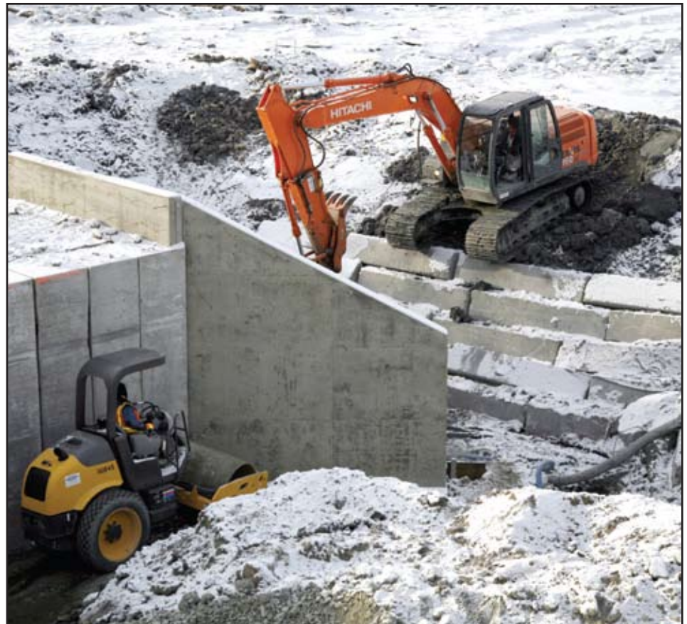
Hamilton Construction finished the job with 10 hours to spare, thanks in part to the reliability of the four Hitachi units on-site.
