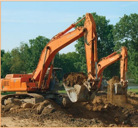
Hitachi machines are extremely fuel-efficient, which keeps daily operating costs down. That's very important to a company that uses an average of 5,500 gallons of fuel each day.
